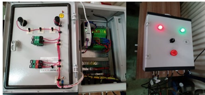
Figure 3. Inner (left) and outer (right) picture of the control panel.
